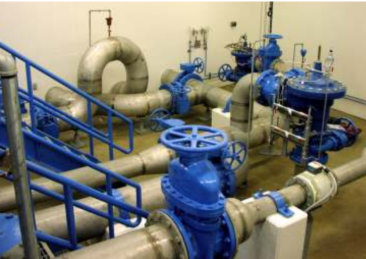
Photo Piping/interior of the chlorination station
