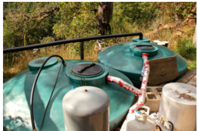
Figure 2: Dual tank with aeration, seasonal irrigation pumps, well top-up, and potable water emergency pump. Source: https://eco-sense.ca/tag/rainwater-harvesting/
