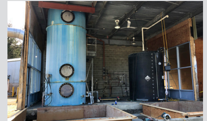
Demolition of the current scrubber building is underway to make space for new scrubber and chemical tanks.
