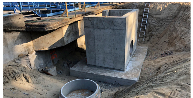
Installation of diversion chamber as part of the new EQ basin project
