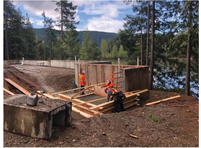
Raw Water Pump Station: Electrical Infrastructure Platform - Foundation Wall
