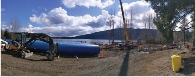
Raw Water Pump Station Site: Pipe ready to be tunnelled into the lake.
