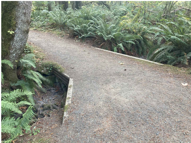
HEADWALL TO BE RAISED TO CREATE BUMPER EDGE SITE PHOTO - SEPTEMBER 2022
