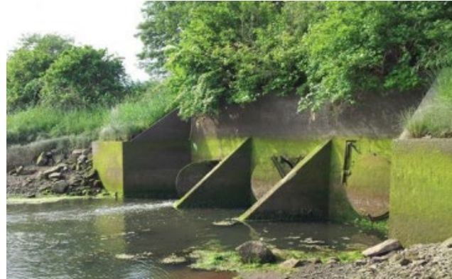
Figure 2-5: Tide gate outlet. Source: CVRD.
