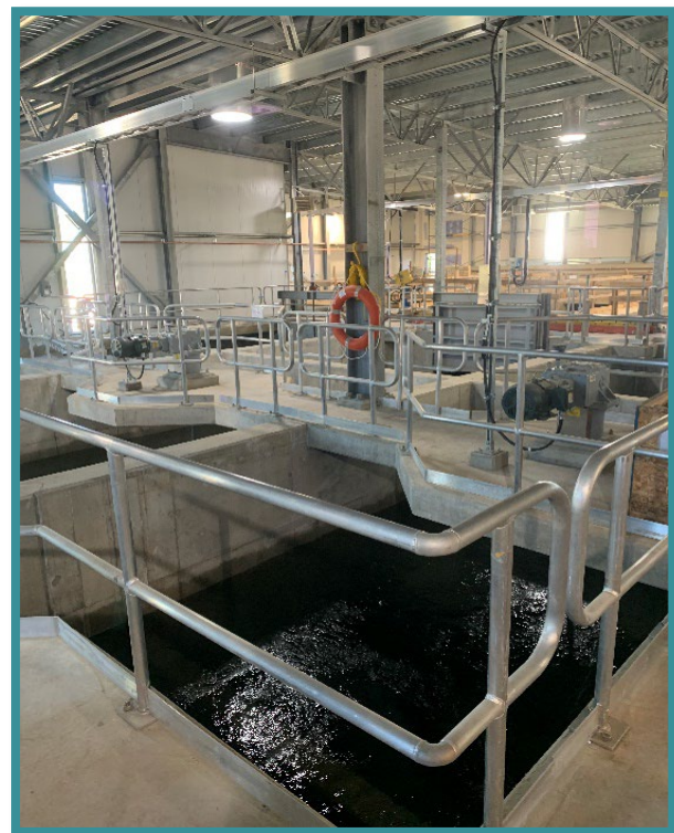
Flocculation tanks and mixing motors.
