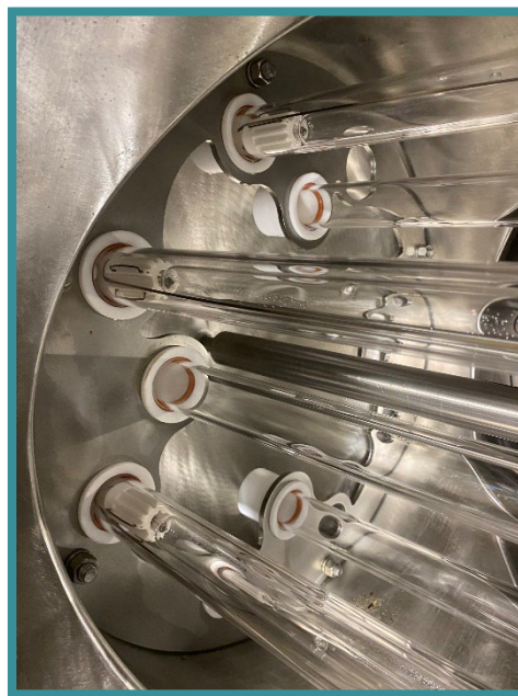
Ultraviolet bulbs inside a reactor.
