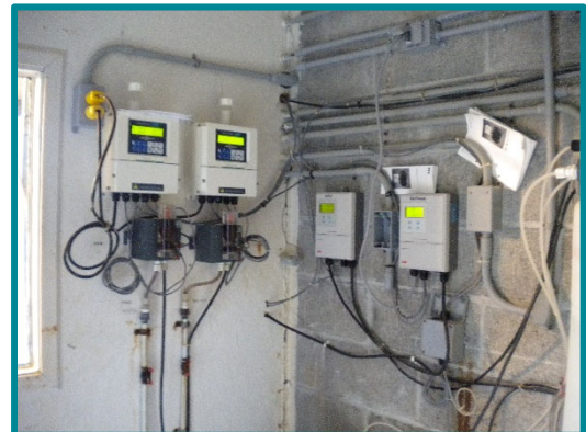
Figure No.2: Chlorine Injection at the Royston Chlorination Station.
