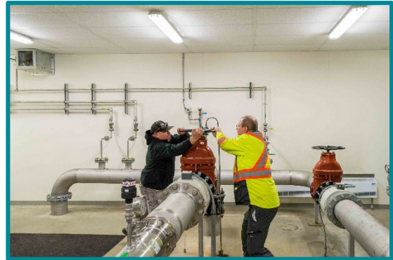
Figure No.2: Closing Valve within BCOB Treatment Facility
