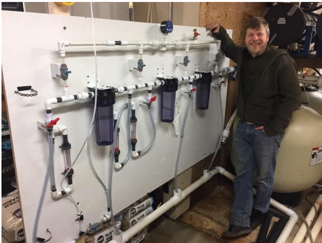
Figure 2: Pilot System Installed in GLID WTP (with IX Column removed for storage)
