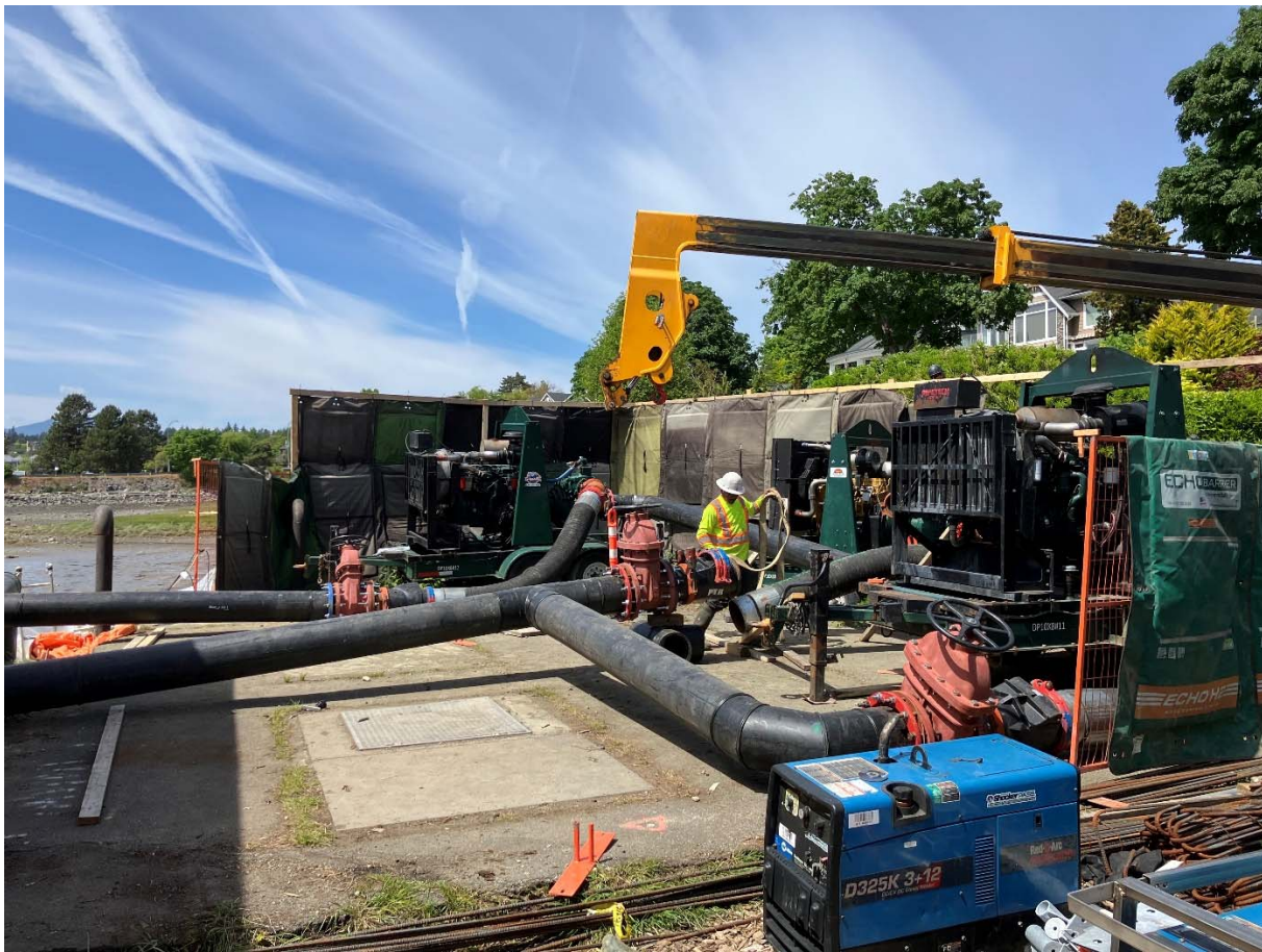
Figure 2 - Bypass Pumping System, Pumps
