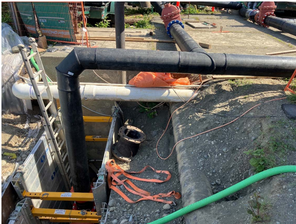
Figure 4 - Bypass Pumping System, Connection to Forcemain
