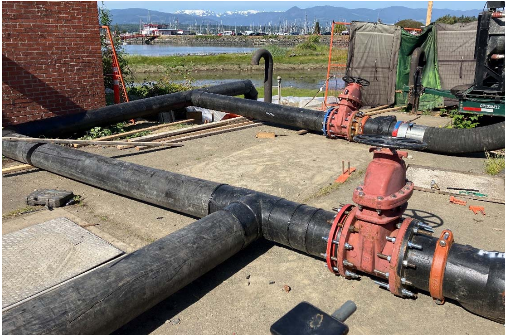
Figure 3 - Bypass Pumping System, Discharge Piping
