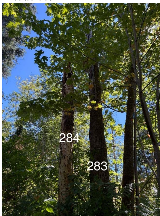
Photo 4. Trees #283 and #284 – Severely decayed stems. Tree #283 (maple) has a failed top and a deep longitudinal crack between stems, while Tree #284 (grand fir) is punky with cavity potential but nearing collapse.
