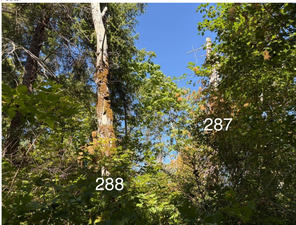
Photo 2. Trees #287 and #288 –Tree #287 (Douglas-fir) is spongy with no cavity value, while Tree #288 (bigleaf maple) is structurally compromised. Both present risk depending on proximity to targets.
