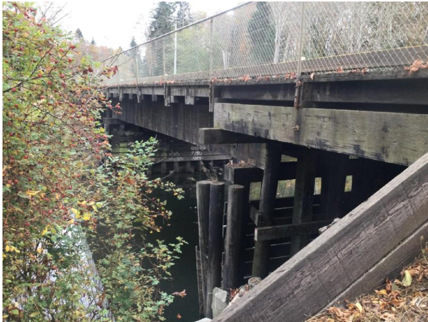
Photo 5. Trent River bridge, view looking south at Highway 19A crossing the river. The Trent River is the largest watercourse that crosses the proposed SES alignment.
